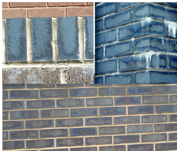
Iridescent appearance caused by light diffraction through fine cementitious material that has leached from mortar.
