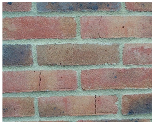
Fire-cracks in clay brick. Cracks do not extend into the mortar joint suggesting their presence when built in.
