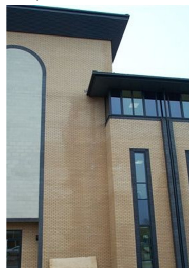
Design detailing has caused saturation staining where water runs off roof ledges.
