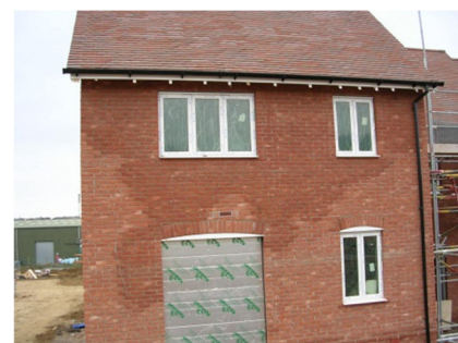
Saturation occurring prior to roof & window placement.
