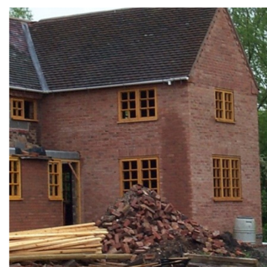
Saturation occurring where downpipes have not been installed.
